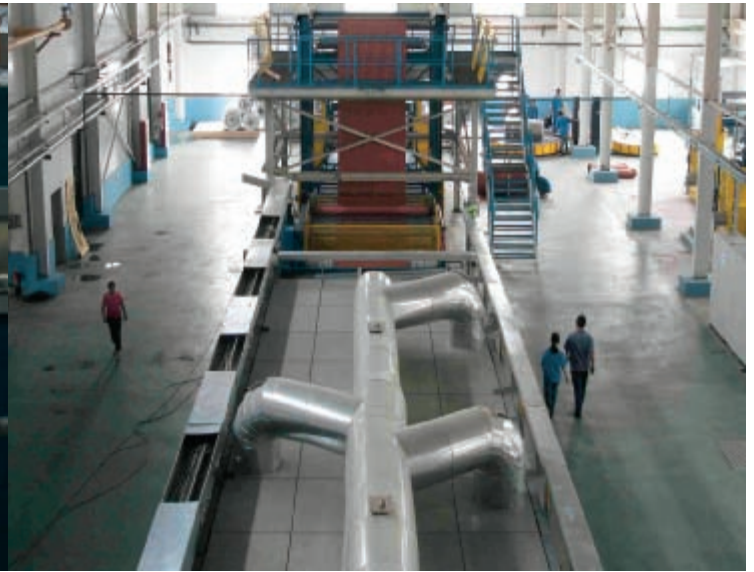
Stenter frame with central exhaust system
