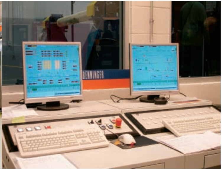
Central process control system
