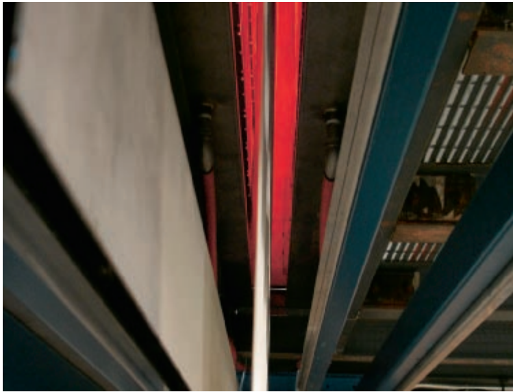
Infrared pre-drier inlet
