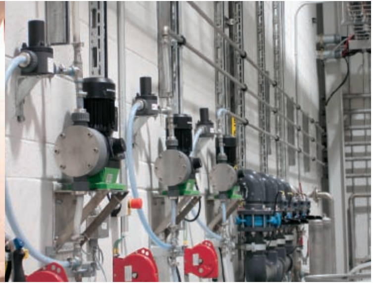
Pumping and piping system
