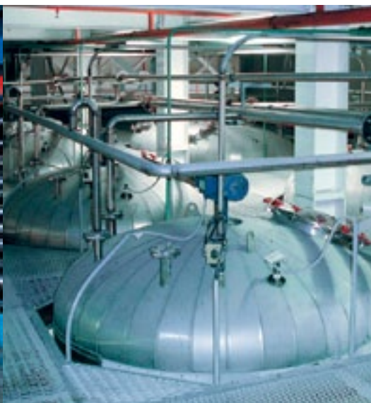
Impregnation solution preparation station
