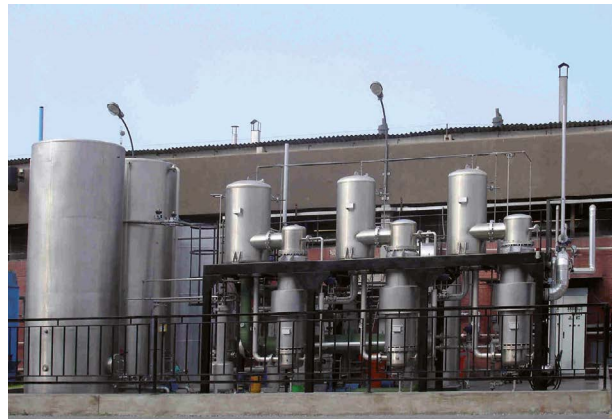
Three-stage lye recovery system
