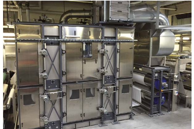
Heat recovery system
