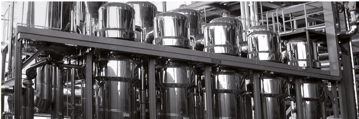
Five-stage lye recovery system
